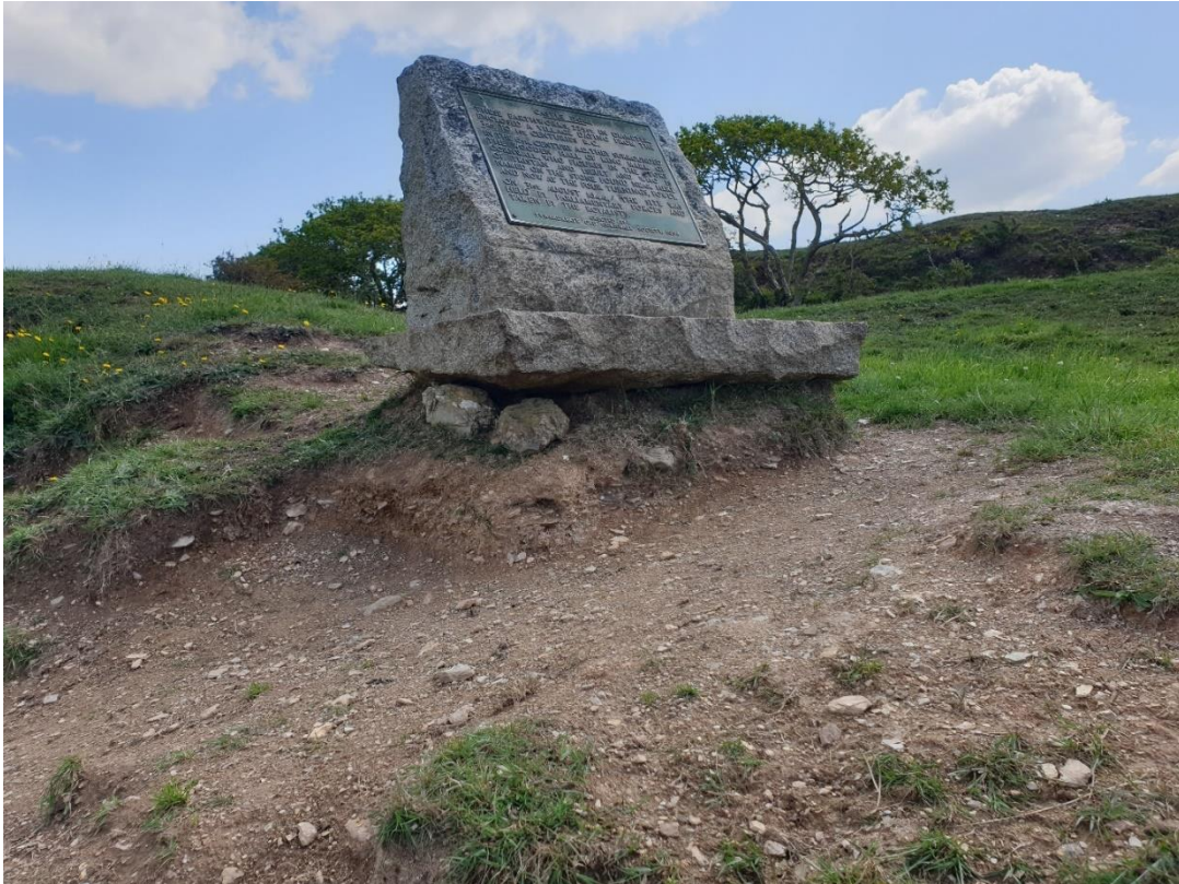
Fig 13 Priority erosion area P3, illustrating the precarious situation of the stone plinth and a recent attempt to support with stones.
