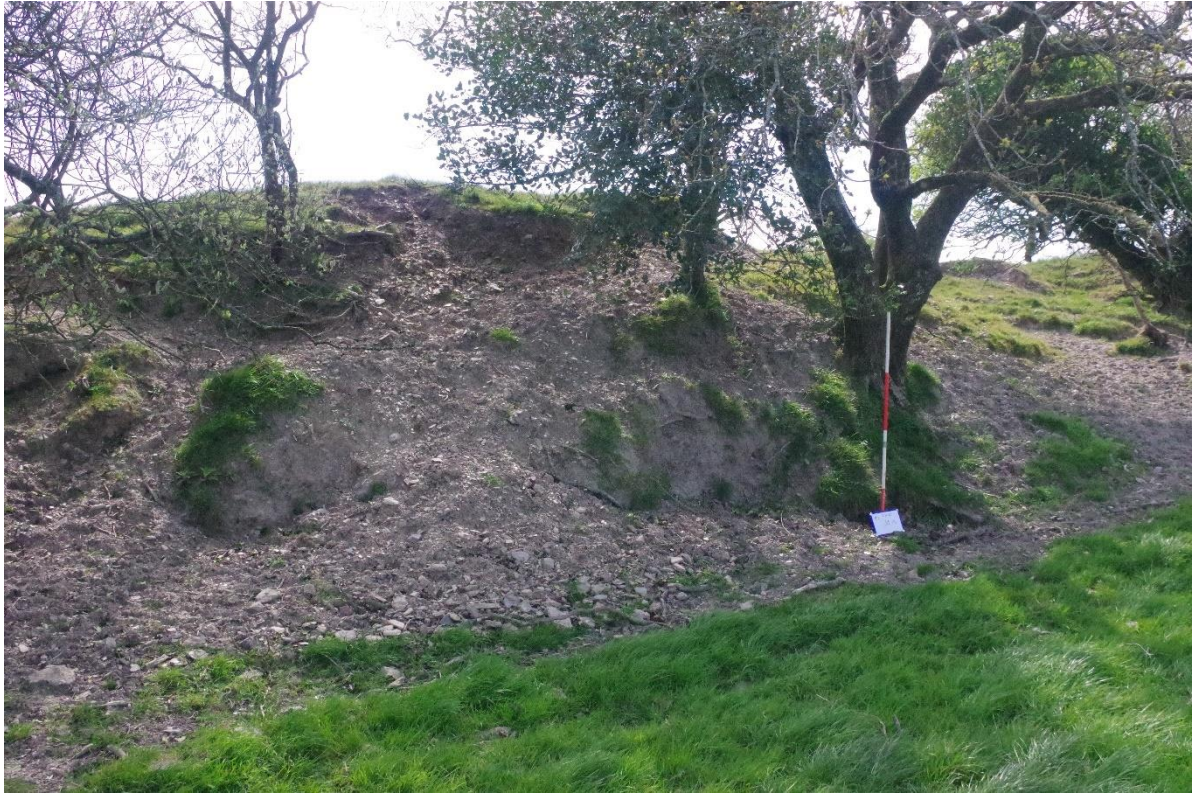
Fig 9 Priority erosion area P2 facing south showing the extent of damage.
