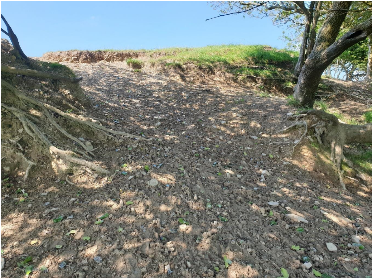
Fig 8 Priority erosion area P2 facing upslope over the outer rampart, showing exposure of tree roots.
